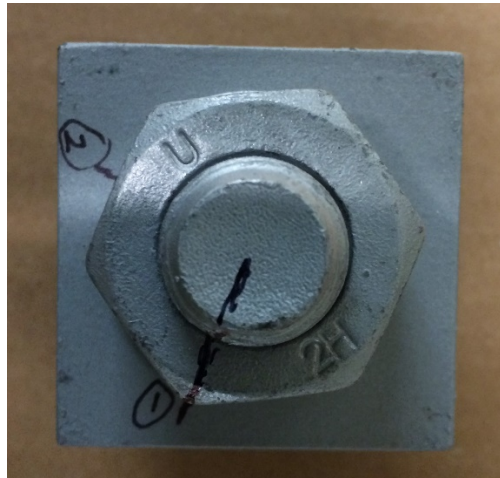
Figure 14 – illustration showing markings for rotation of nuts from snug tight starting position (1) to 1/3 turn + 30° (150° total) beyond snug (2).
